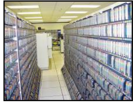
OCIO tape storage area BEFORE new tape storage project.
